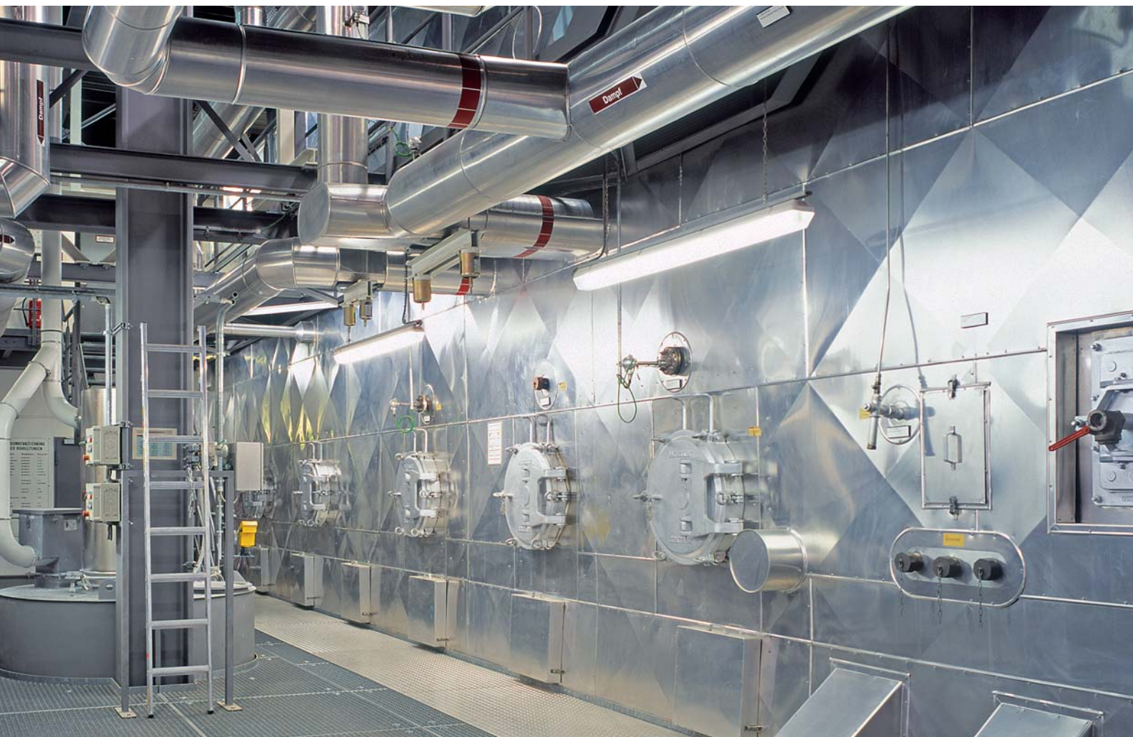
The boiler room of the incineration plant. In the two boiler lines, exhaust air with 860°C from the sludge burning process heats up water-filled tubes thusly generating a high pressure steam with 400°C and 40 bars. The steam first propels a power turbine and is then used for heating the sludge driers.
