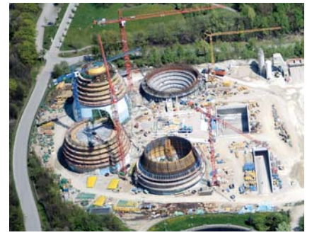
When finished, the digesters will extend 31.5 metres above and 13.5 metres below ground level.
