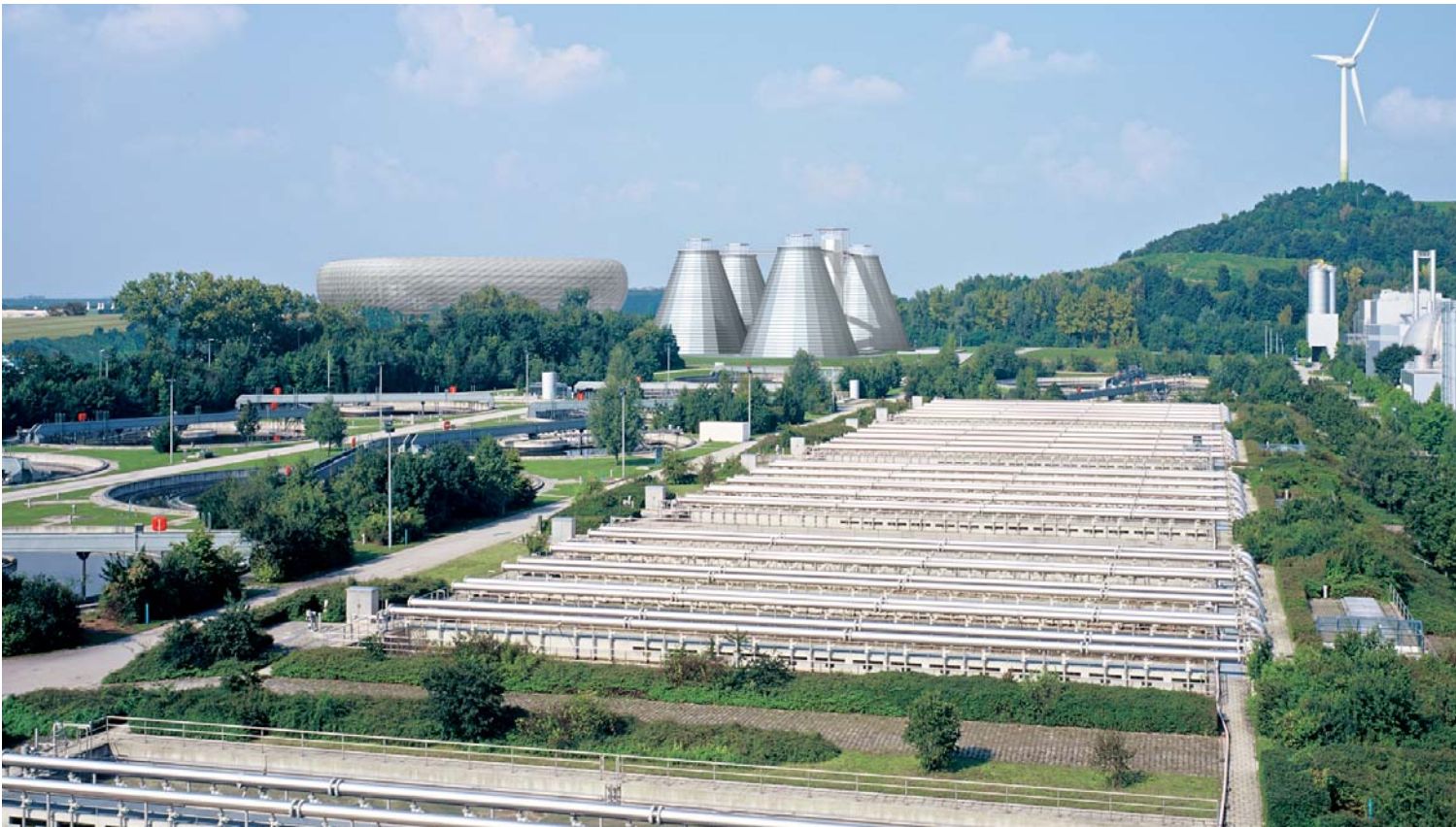
The second biological treatment stage: The new sludge digesters (here still pictured as a simulation).
