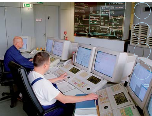
Incineration plant control room: From here the burning process of waste sludge from the two treatment plants is controlled and monitored.
