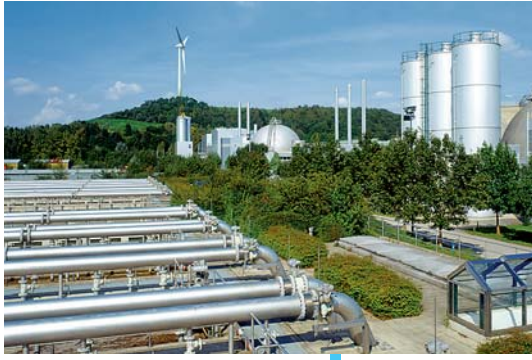
Wastewater Treatment Plant Gut Großlappen
